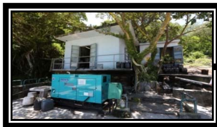
Existing Government-owned Diesel Generators
